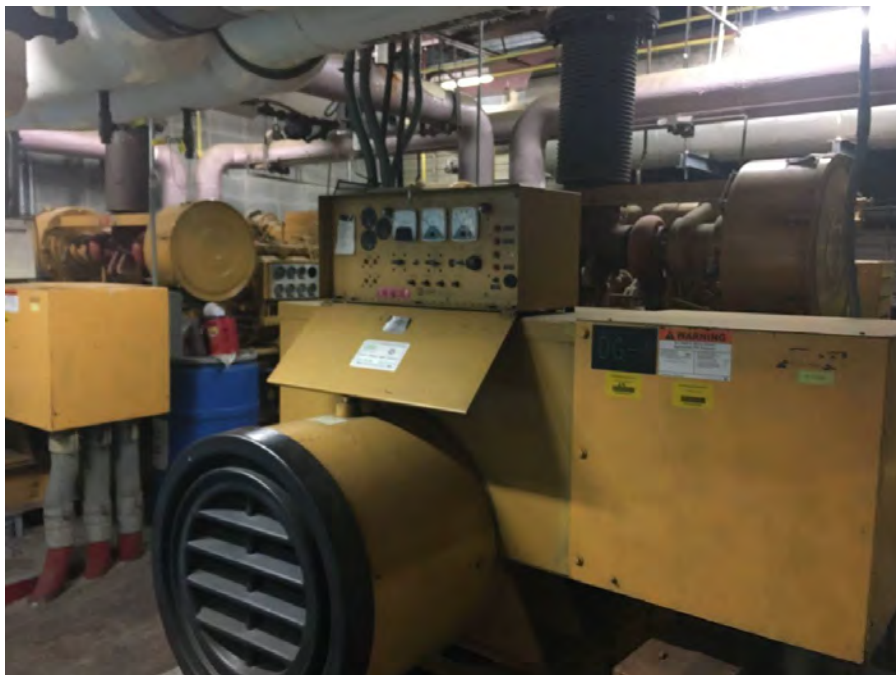
Figure 39 Muirkirk Road Complex - Existing Out-Dated Generators
