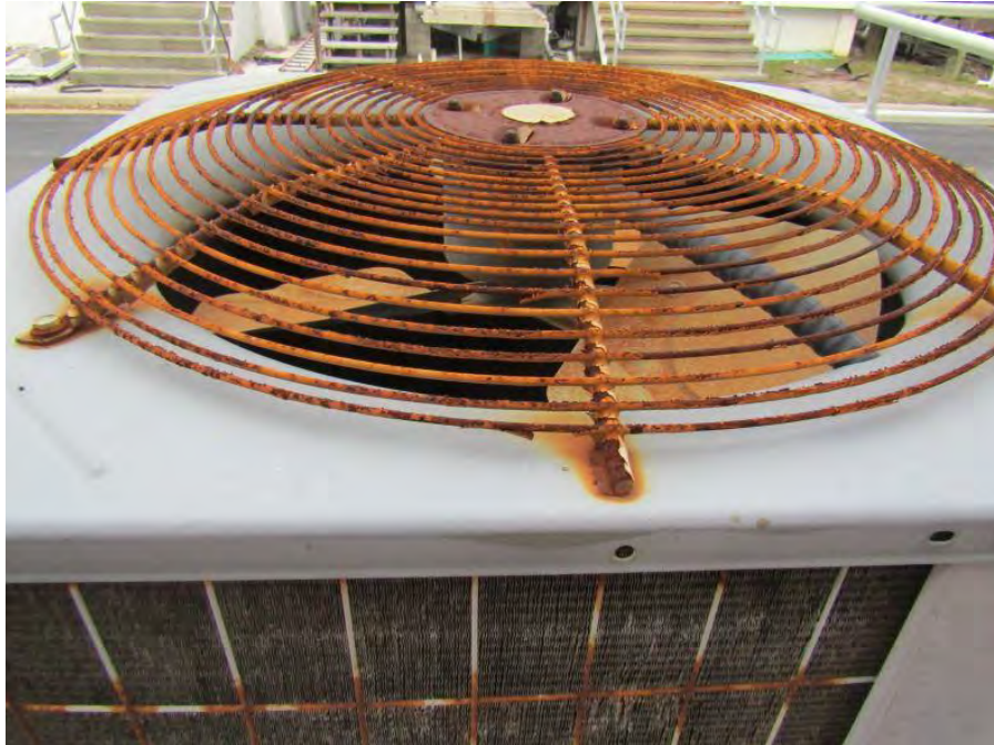
Figure 33 Gulf Coast Seafood Laboratory - Existing Air Conditioning Unit
