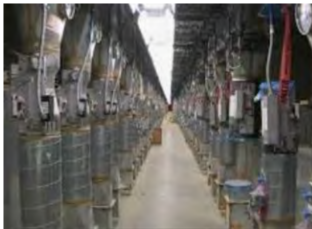
Figure 30 State-of-the-Art White Oak Infrastructure: Advanced Air Terminal Units Supporting Laboratories
