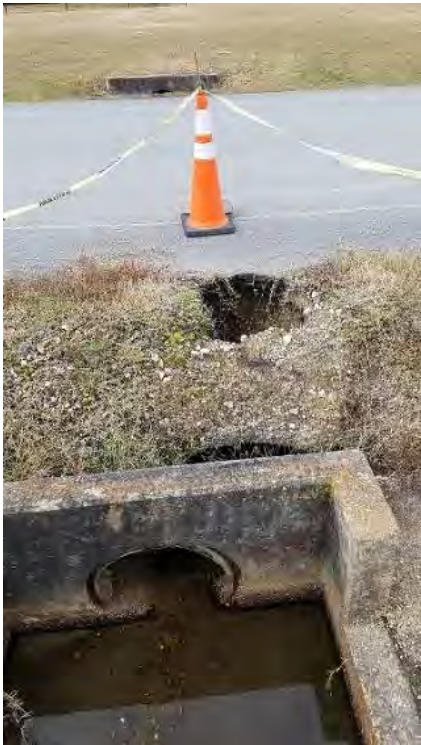
Figure 36 Jefferson Labs Drainage Infrastructure
