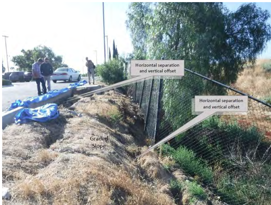
Figure 40 Pacific Regional Laboratory Southwest - Soil Settlement Issues
